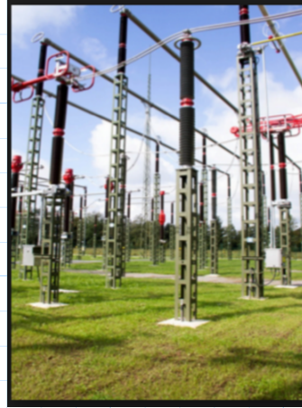
Picture of post insulator; stacks of insulators mounted on a post
