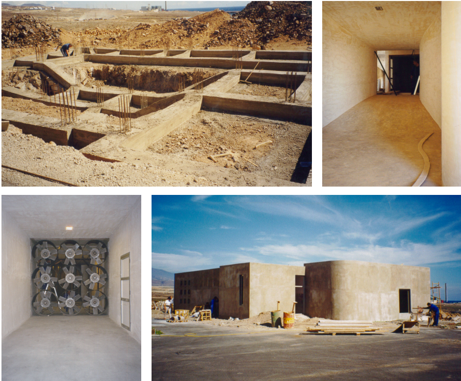
Figure 15. Photographic sequence of the construction of the ITER Low Speed Wind Tunnel. The top left picture shows the foundations, the top right the contraction, the bottom left the power plant and the bottom right a view from the outside almost at the end of the construction.
